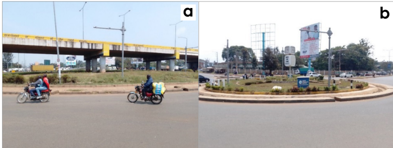
Figure 12a: Kondele Roundabout done through PPP. Current status: unkempt, untidy and vandalized
