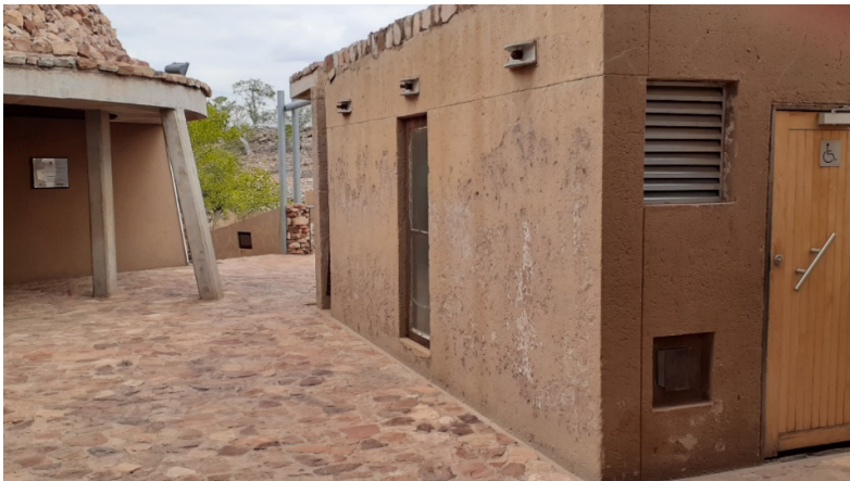
Figure 10: Mapungubwe Interpretation Centre wall requiring maintenance Source: Image taken by author
