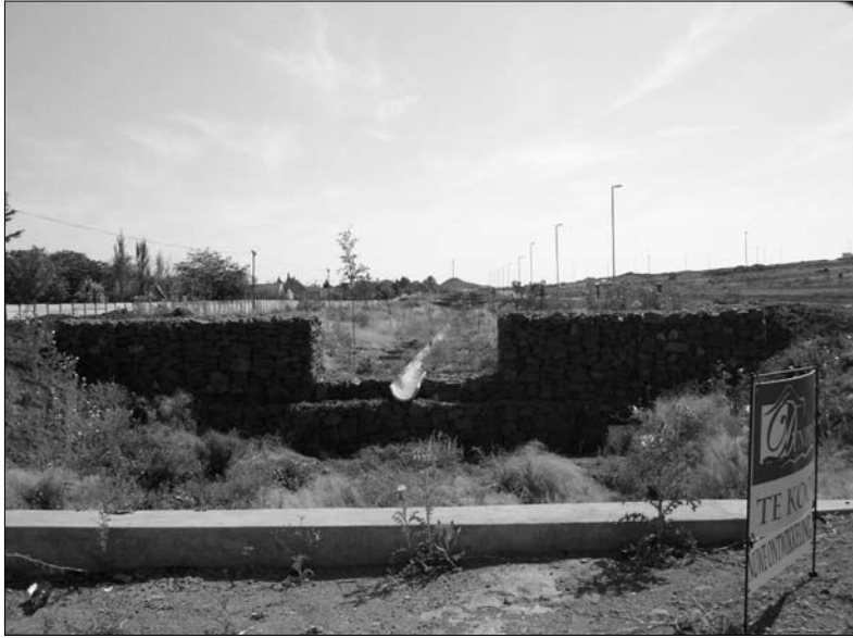
Figure 5: Storm water canal used as a dumpsite Source: Steyn & Schoeman 2006: CD-ROM
