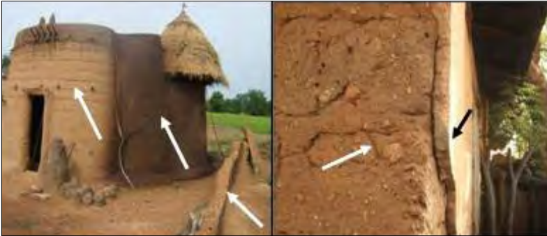
Figure 15: Traditional earthen buildings deterioration due to water penetration showing the urgent need for wall coatings in Benin
